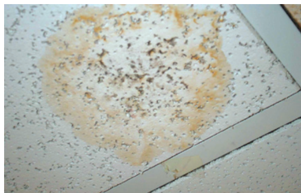
Water damaged ceiling tile with fungal growth
